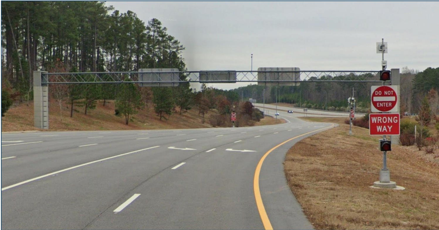
Proprietary Wrong-Way Detection System at Davis Drive and I-540
